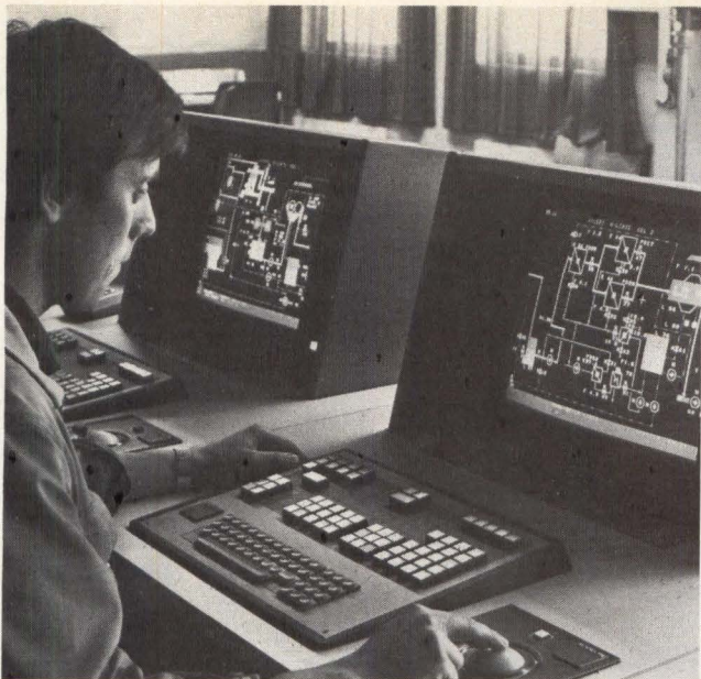
Fig 3 Operator communications units at control room. Each of four consoles contains color CRT display, display processor, terminal controller, function and alphanumeric keyboards, and trackball. Operator calls for diagrammatic display through commands on function keyboard and chooses area for study by moving trackball. Alphanumeric keyboard enables plain language communication
